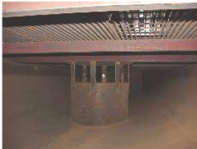
Typical location of FAC at bottom of heater shell
